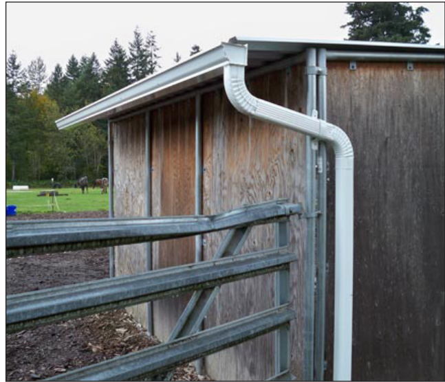
Figure 13. A roof runoff structure like the one pictured helps collect, control, and transport precipitation from roofs. Photo courtesy of the King Conservation District.
